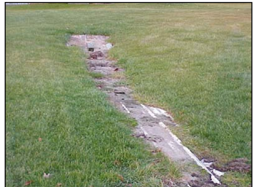
Failing POWTS, rural Clark County
